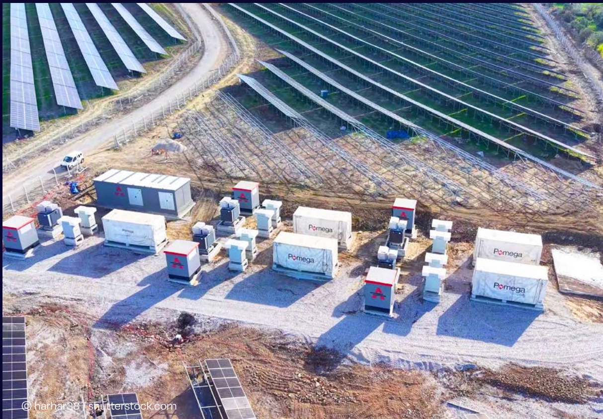
Battery Energy Storage System (BESS) installed alongside solar farm, Aliğa, Türkiye
