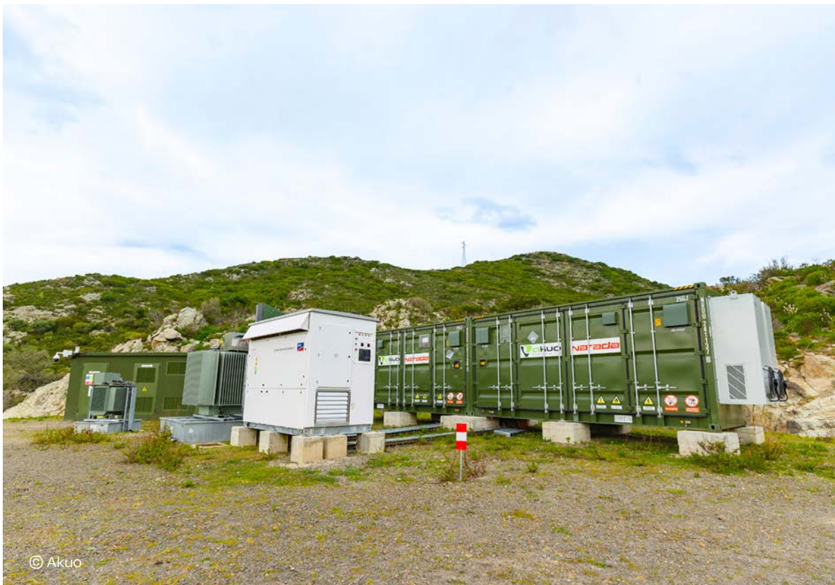
Murellu, Pieve, Corsica, France — 1.7 MW solar PV with 5.2 MWh battery storage
