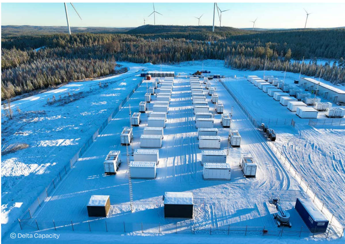
Ånge Energy Storage, Ånge, Sweden — 70 MW / 160 MWh battery energy storage system
