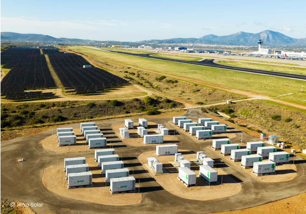
Athens International Airport, Athens, Greece — 51.5 MW solar PV with 82 MWh battery storage
