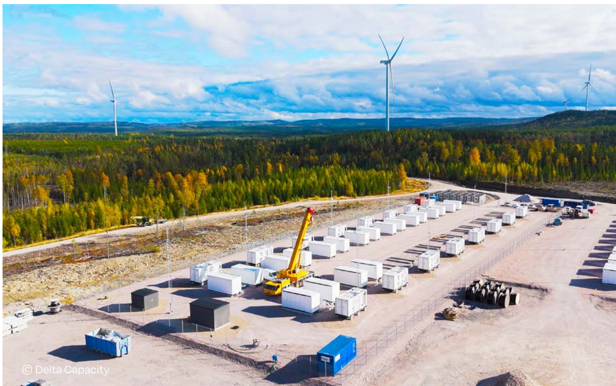
Ånge Energy Storage, Ånge, Sweden — 70 MW / 160 MWh battery energy storage system
