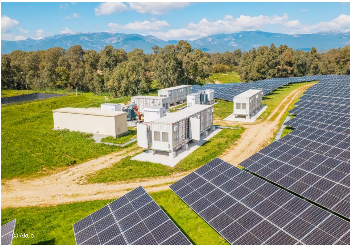
Capu di Padula, Porto-Vecchio, Corsica, France — 5.08 MW solar PV with 16.1–16.3 MWh battery storage
