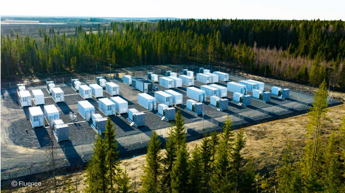
Uusnivala battery project, Nivala, Finland - 55 MW / 110 MWh battery storage project
